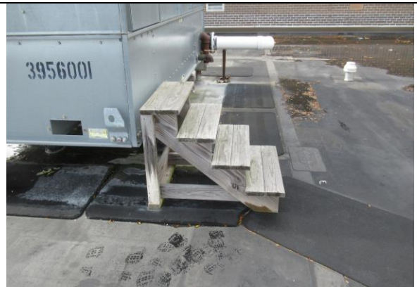
Existing HVAC Equipment Service Stairs And Walkway System Require Replacement.
