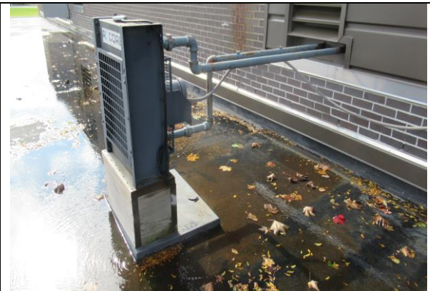
HVAC Equipment Requires Proper Support Component
