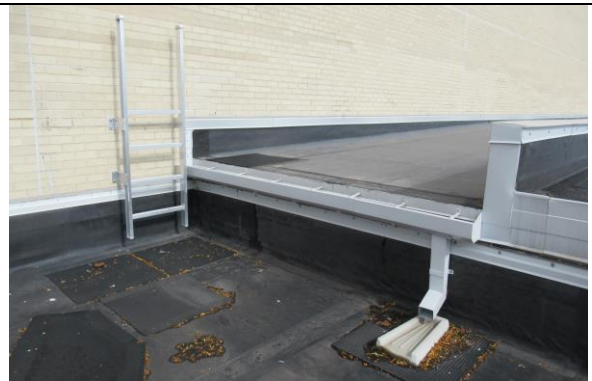
Existing Wall Mounted Roof Access Ladder And Downspout Require Modifications To Accommodate Tapered Rigid Insulation System.
