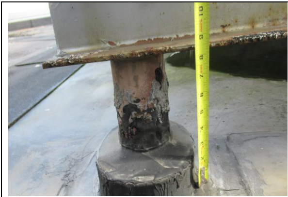
Mechanical Equipment Supports May Need To Be Raised To Comply With Manufacturers' Recommended Minimum Flashing Height, Depending Upon Roof System Drainage Design. Raising The Height Of The Equipment Supports Would Require Disconnection, Modification, Reconnection And Testing Of The Process Piping, Electrical And Control Wiring.
