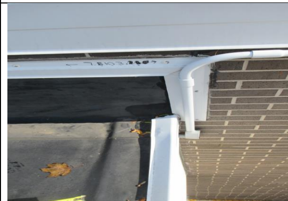
Existing Wall Mounted Electrical Supply Requires Modifications To Perform The Work.
