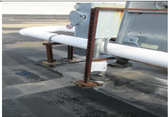
Existing Pipe Supports Require Replacement.
