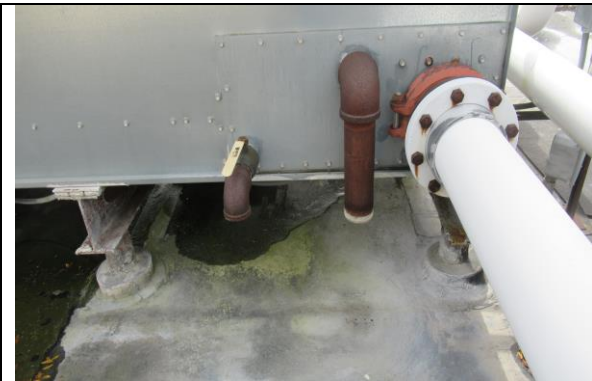
Existing HVAC Equipment Drains Require Plumbing Extensions To Direct Water Discharge To Internal Roof Drain(s).
